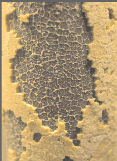
Lime precipitation in the boiler
